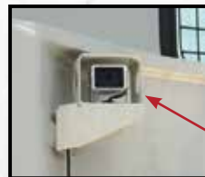
Integrated air conditioning
